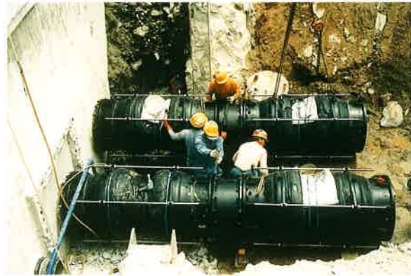
DN700mm WUU-type Subsidence 1000mm
