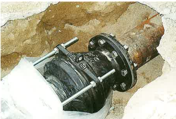
Hong Kong (TSEUNG KWAN O AREA) DN150mm WFF-type Subsidence 300mm
