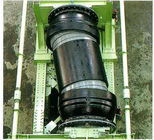
Inspecting watertightness of TAI-FLEX at subsiding. Watertightness test for subsidence and repeating test for subsidence DN1200mm
