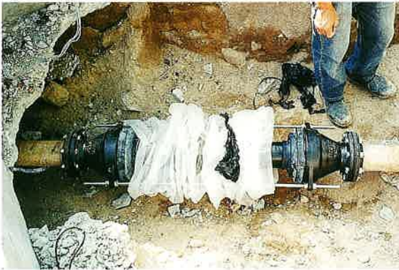
Hong Kong (TSEUNG KWAN O AREA) DN100mm WFF-type Subsidence 300mm
