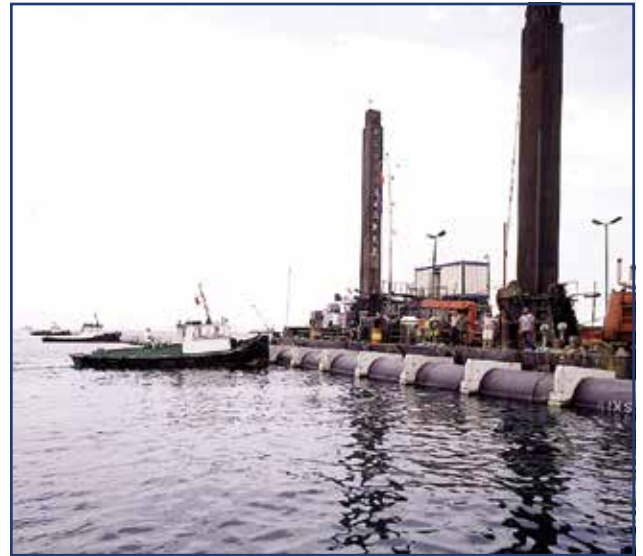
Picture 1.1.2a - A view from sea discharge application of 1600 mm o.d. PN 4 PE pipes in Istanbul.
